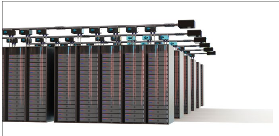
'Hot Aisle Cold Aisle' Arrangement
